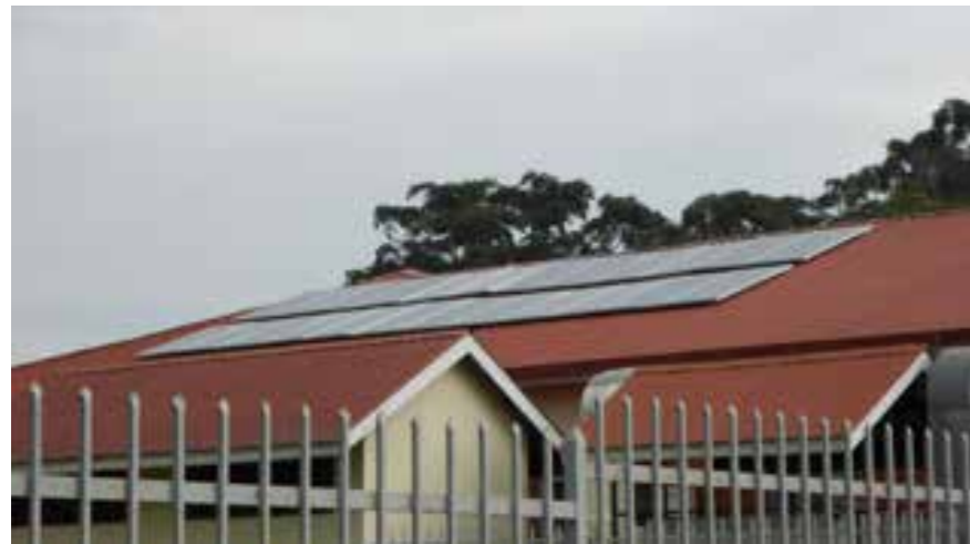
5c PV-Anlage Kamuli Mission Hospital
