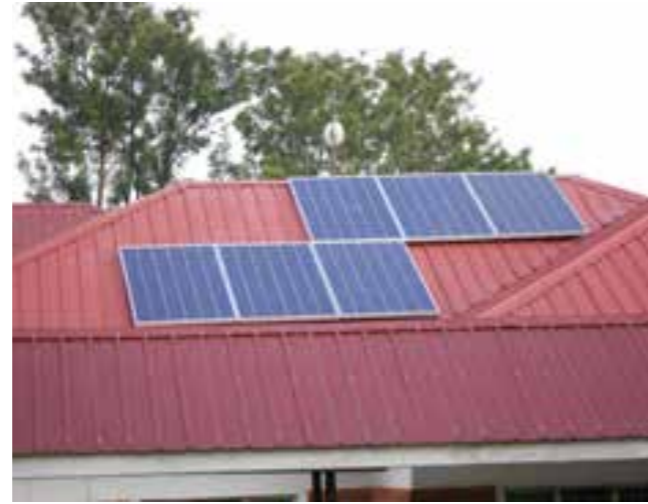
5b PV-Anlage Kamuli Mission Hospital 1
